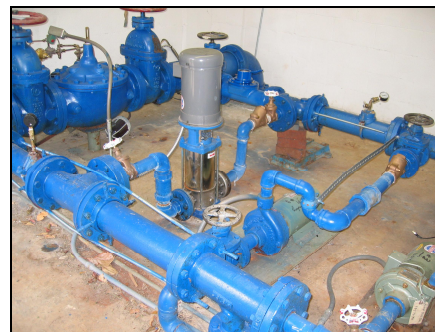
Center Street Booster Pump Station
