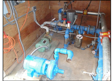
Hilltop Booster Pump Station
