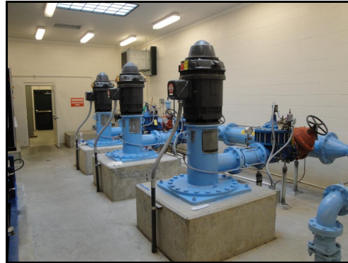
Main Booster Pump Station
