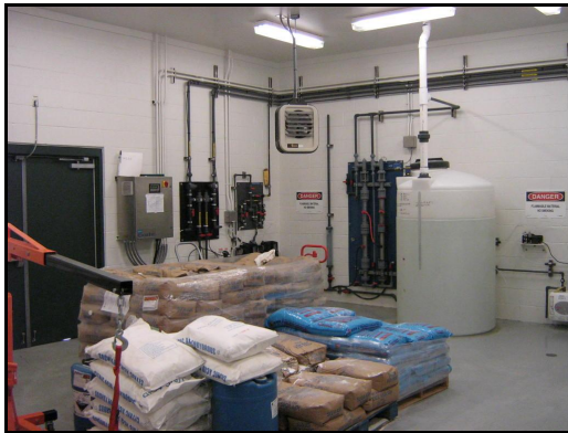
WTF Chlorination Room
